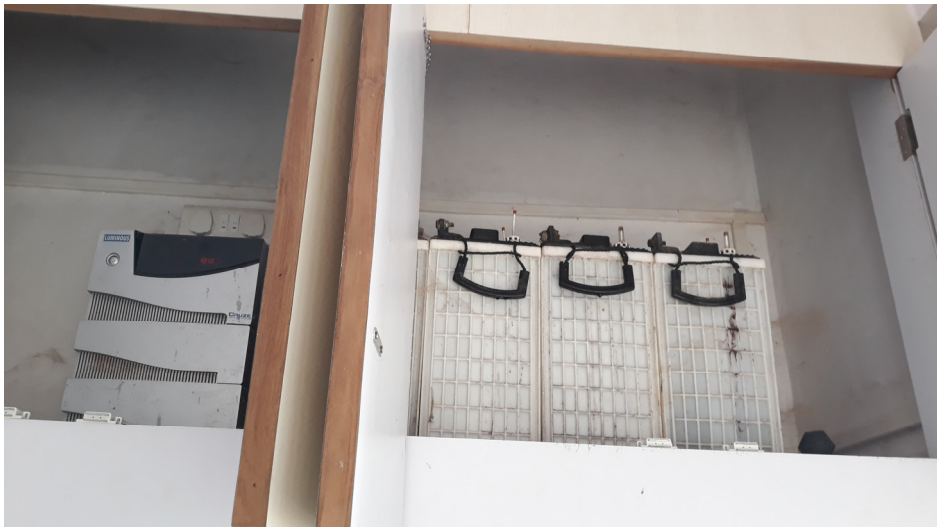
Battery Backup II
