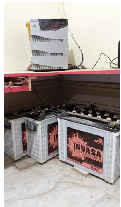
Battery Backup I
